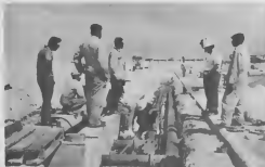
At the valve pit, Project Leader Carlos Bisip (2nd from r) watches final checks being made before closing ditch containing bunker lines at H-Dock in Oranjestad.
